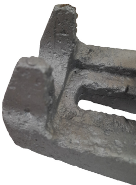
4. Excessive corrosion to casting
